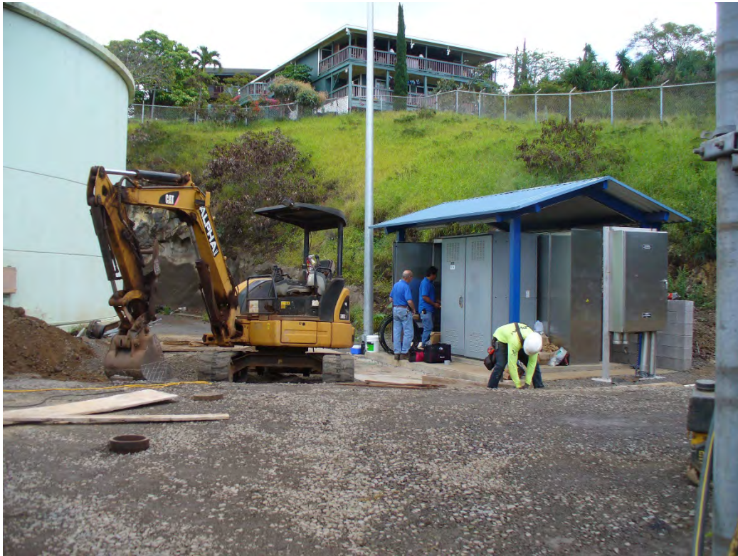
CIP upgrade of new pumps and motor control center at Maui Meadows #18 booster station
