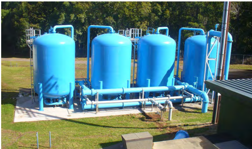
GAC Filters at Pi'iholo WTP
